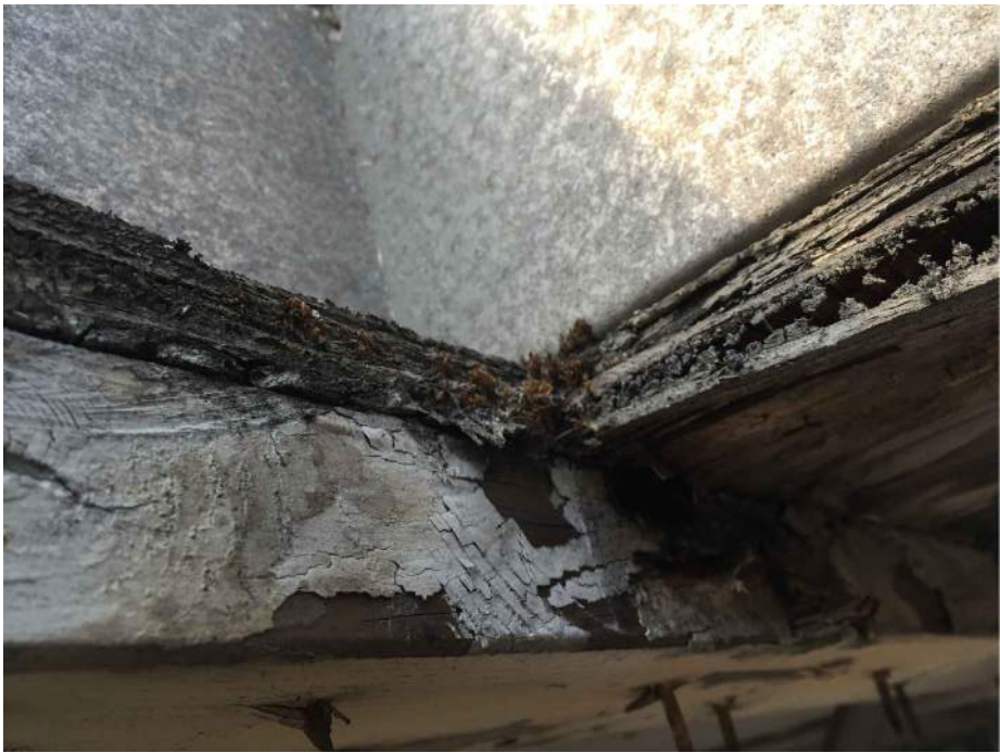
TYPICAL DAMAGE © (E) SKYLIGHT
