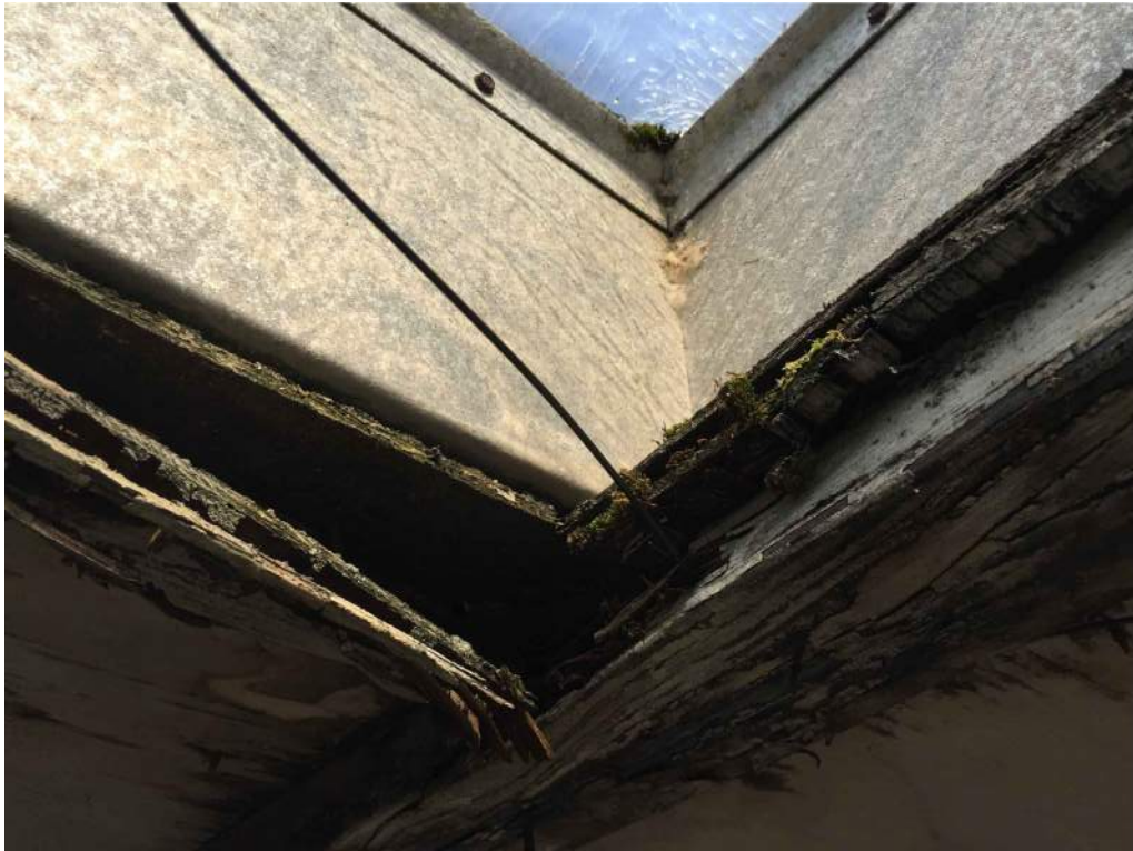
TYPICAL DAMAGE © (E) SKYLIGHT
