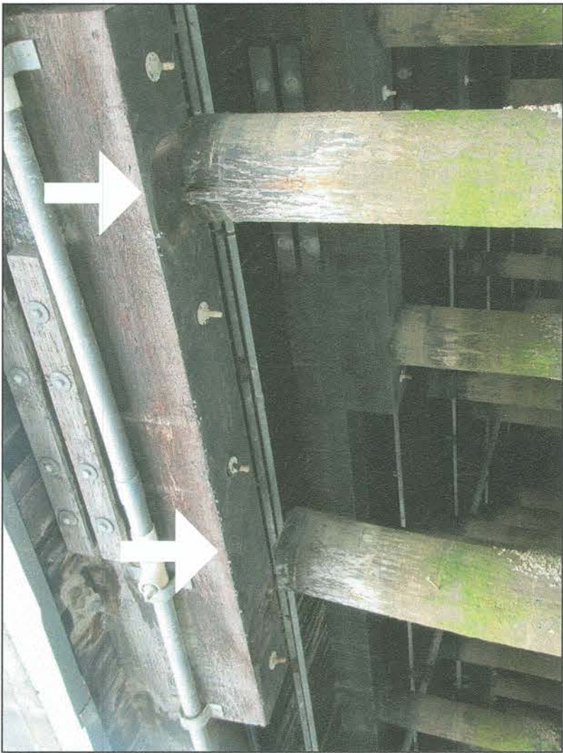
P9 MISALIGNED PILES B112:D & B112:E S3 LOOKING WEST
