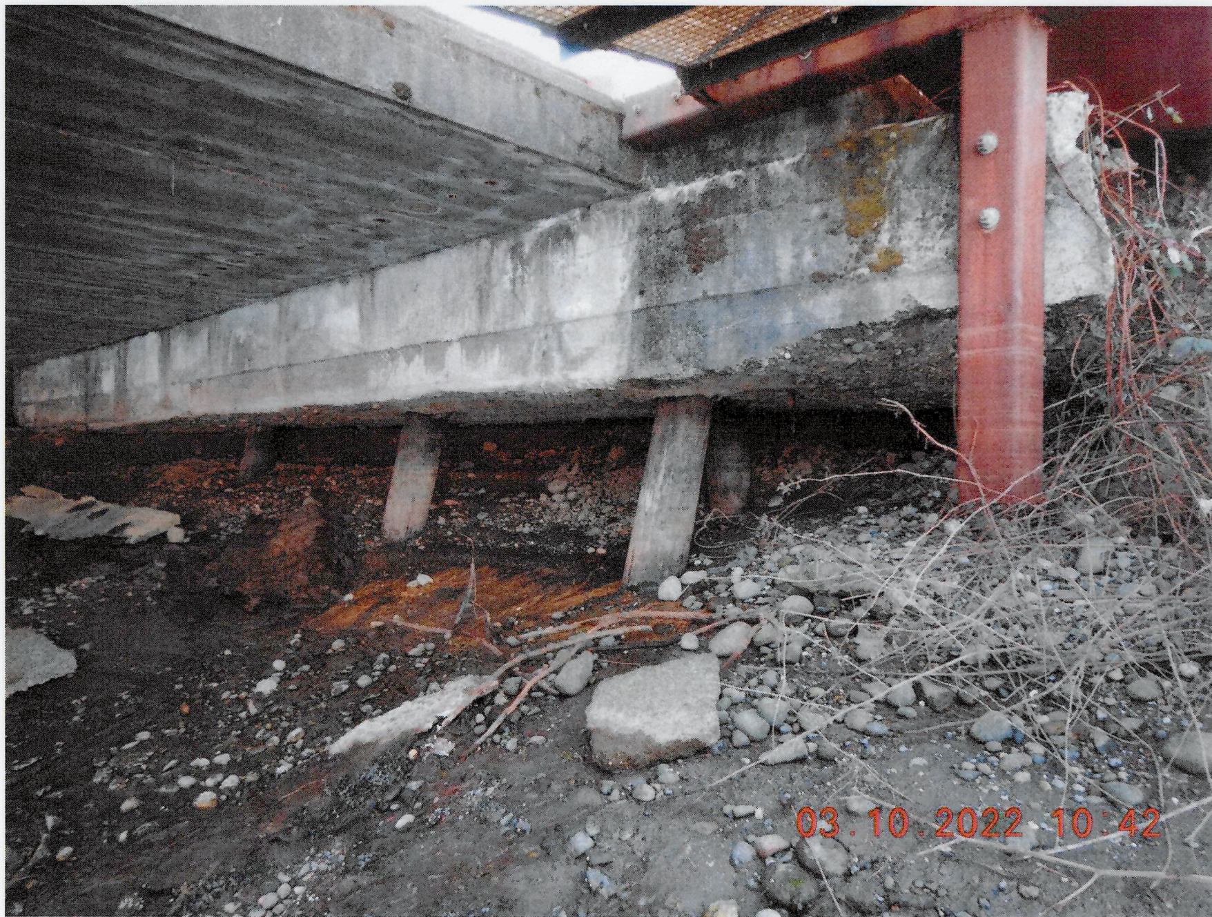
P1 G3 UNDERMINING AT ABUTMENT LOOKING: SOUTH
